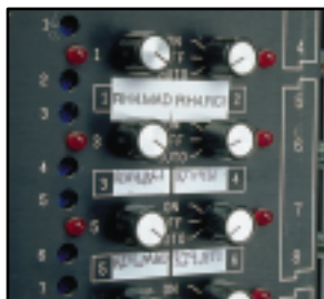
Label switches, relays and other devices
