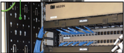
Lacing Panel shown in cabinet
